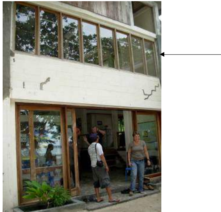
Figure 15. Lumba Lumba dive shop on Pulau Weh (A. Hagan). Note arrow points to line across window indicating tsunami water level (~5 m above sea level) on 26 December 2004.
