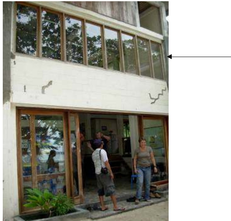
Figure 15. Lumba Lumba dive shop on Pulau Weh (A. Hagan). Note arrow points to line across window indicating tsunami water level (~5 m above sea level) on 26 December 2004.
